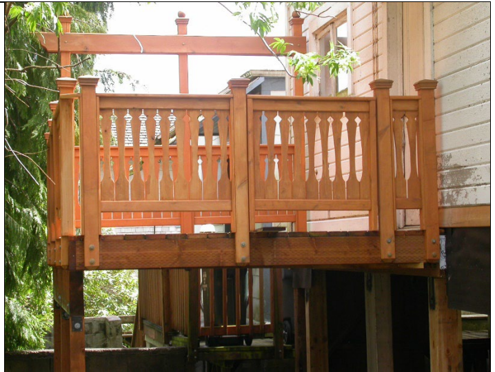
Incorrect: Supports on outside of decking visible/exposed; Open below deck with visible supports.
