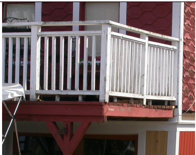
Keep handrails simple and low. An open upper rail can be added to help meet required building codes.
