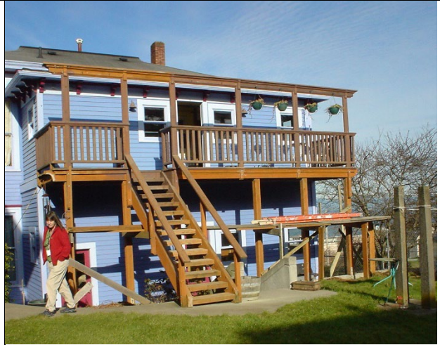
Incorrect: Support posts do not line up between 1 st and 2 nd floors; balusters too tall; handrail extends past post; no spindles along staircase.
